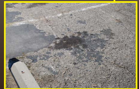
Oil/Grease Spots Saturates then softens the asphalt which leads to decay
