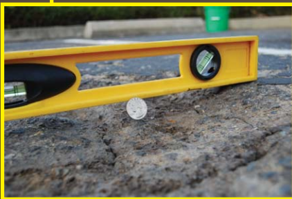
Rutting Another wet season and this may have become a pothole
