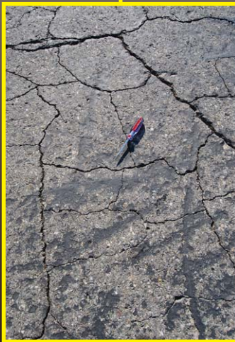
Block Cracks/Alligating Removal & Replacement is usually the only option
